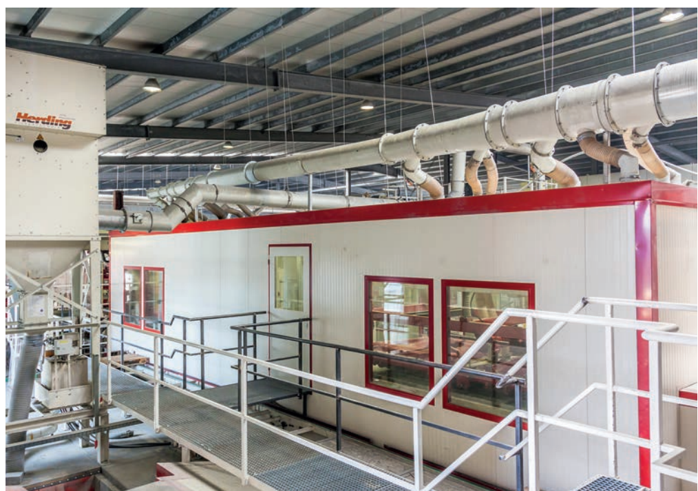
Herding Flex as a central filter plant in use at the Godelmann company
