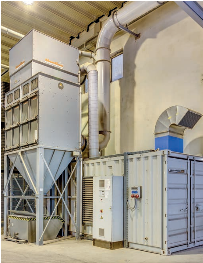
Booth extraction with clean air recirculation into a compressor room
