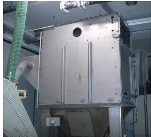
Picture 3: Filter unit
