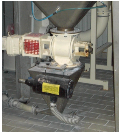
Picture 2: Rotary air lock
